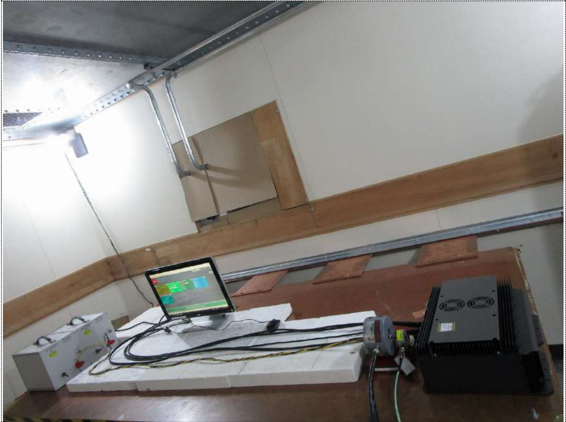
View of Measurement (Power line)
